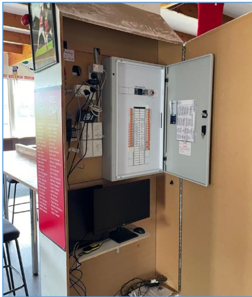
Figure 1: Push the scoreboard fuse switch to the RIGHT (ON)
